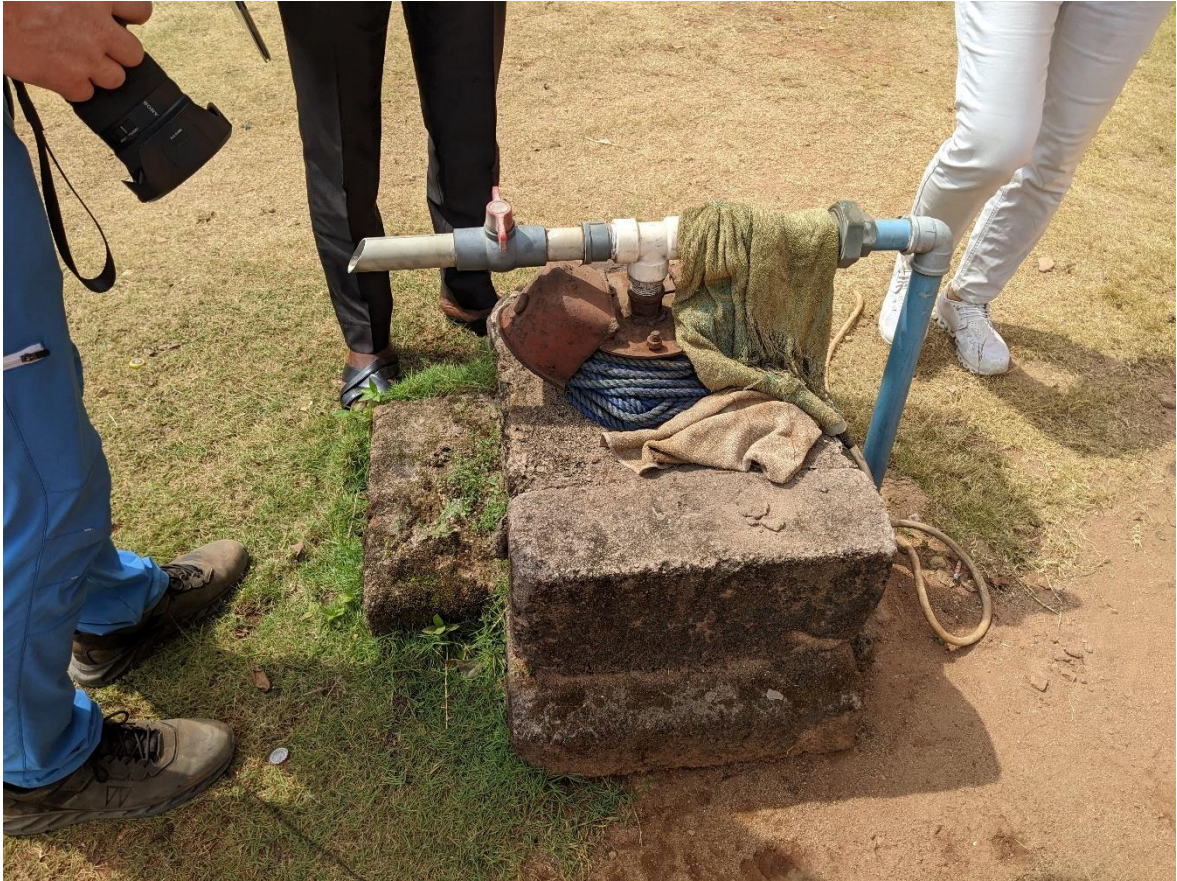
Figure 11 Water supply at the hospital
