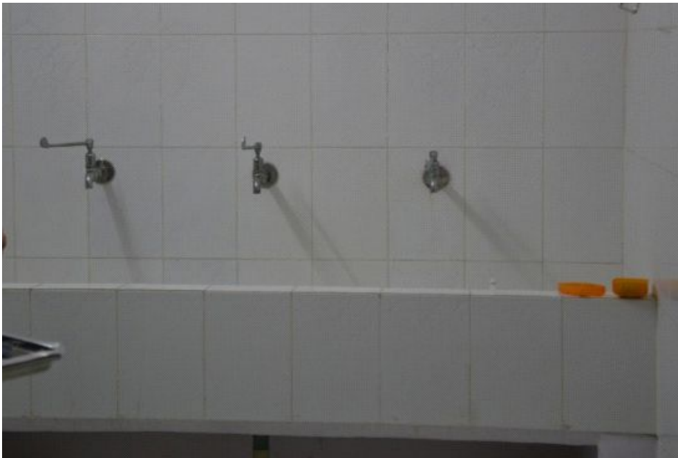
Figure 18: Sample 6: water tap operating theatre, first floor – Photographer: Isabella Dicker
