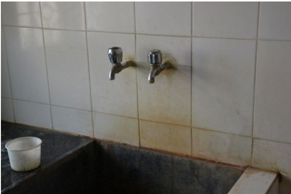
Figure 24: Sample 12: water tap with R.O.-plant water, ground floor – Photographer: Angelika Schirnhofner
