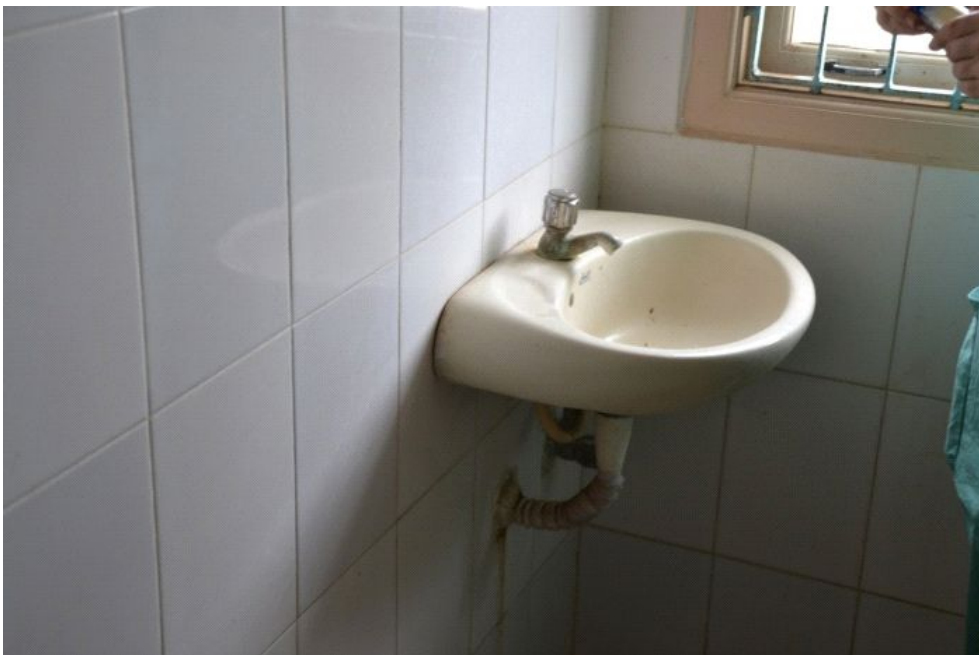
Figure 22: Sample 10: water tap room D, ground floor – Photographer: Angelika Schirnhofner
