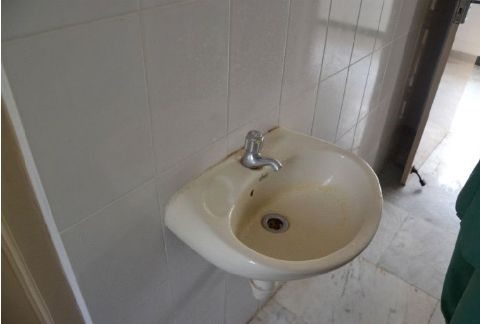
Figure 19: Sample 7: water tap ICU, first floor – Photographer: Angelika Schirnhofner
